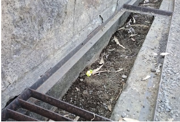
Accumulation of sediment or debris in drainage structures.
