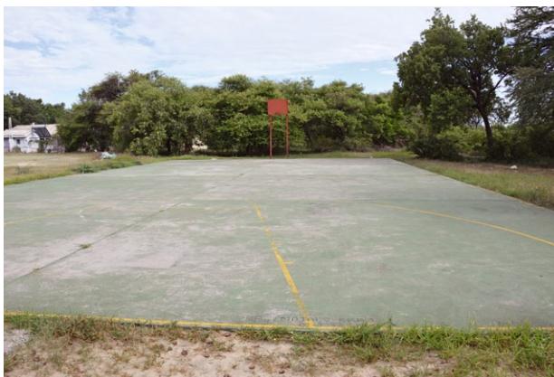
Faded line marking on Basketball court.
