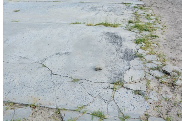
b) Weathered and cracked surface conditions and lack of proper cleaning and maintenance.
